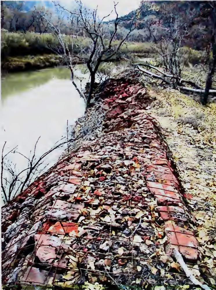
FIGURE 2. Rock and wire revetments channelize the Virgin River in Zion National Park.
