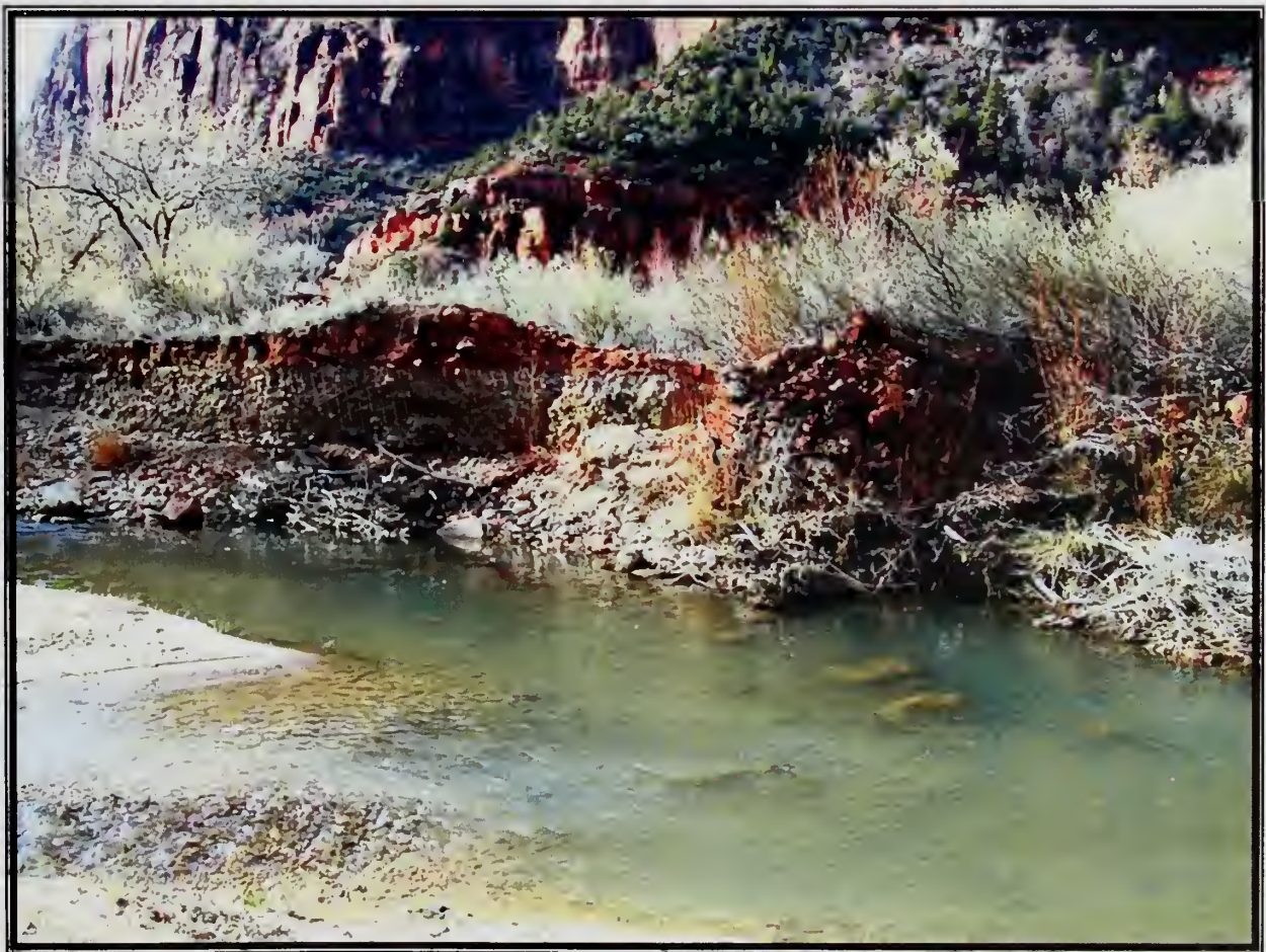
FIGURE 20. Rock revetments in disrepair near Zion Lodge
